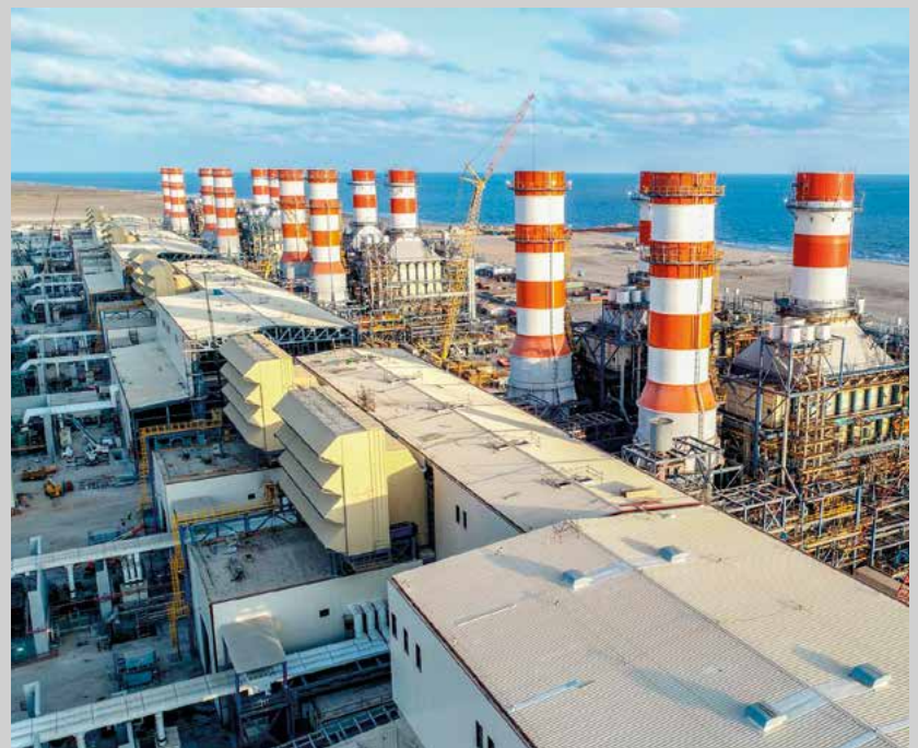
Combined Cycle Power Plant (CCPP) in Beni Suef, Egypt
